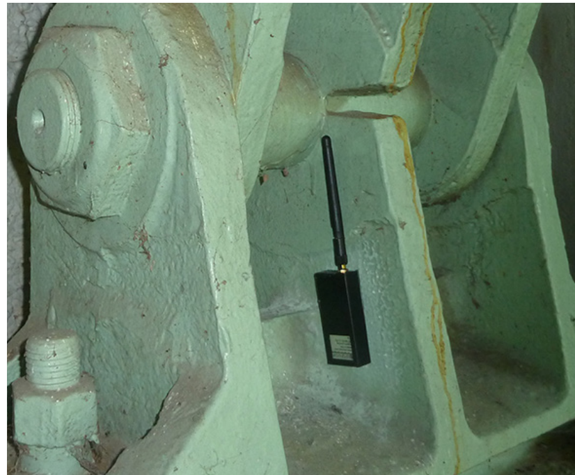
Resensys structural stress monitors are mounted beneath bridge trusses and other hard-to-access locations. These monitors require ultra-long-life bobbin-type \text{LiSOCl}_2 batteries to minimize the need for costly and dangerous battery replacements.
